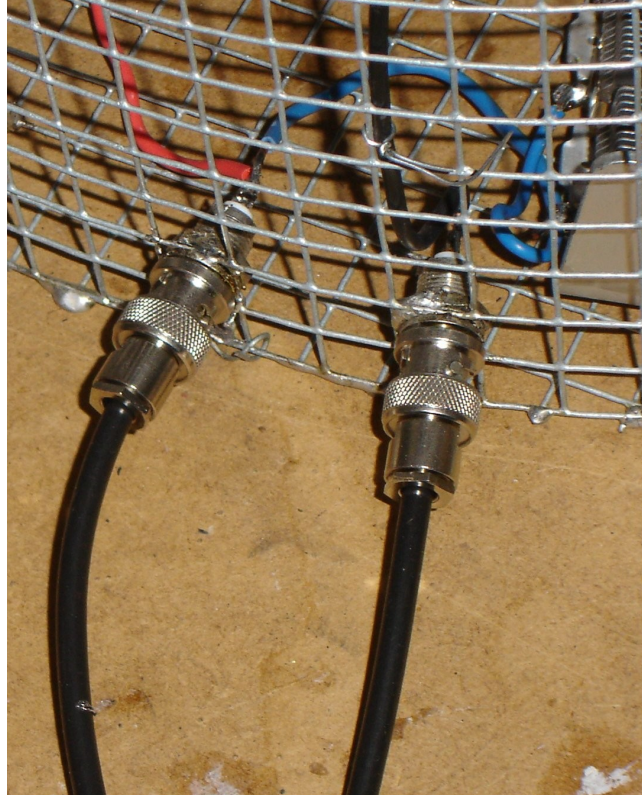
Figure 26: Coaxial cable entry points through the mesh using BNC connectors.
